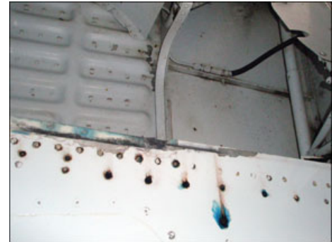
One sore spot with owners is sealing the integral fuel tanks in each wing. At left are the underlying fuel stains and corrosion resulting when repairs are left too long.
